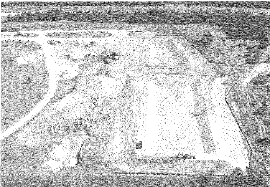
Chromium sludge was completely removed from two containment ponds at the U.S. Department of Energy's Portsmouth Gaseous Diffusion Plant, detoxified, and placed in these specially-built monocells located at the plant's sanitary landfill. Completion of this project marks a significant phase in environmental recovery at the plant.
